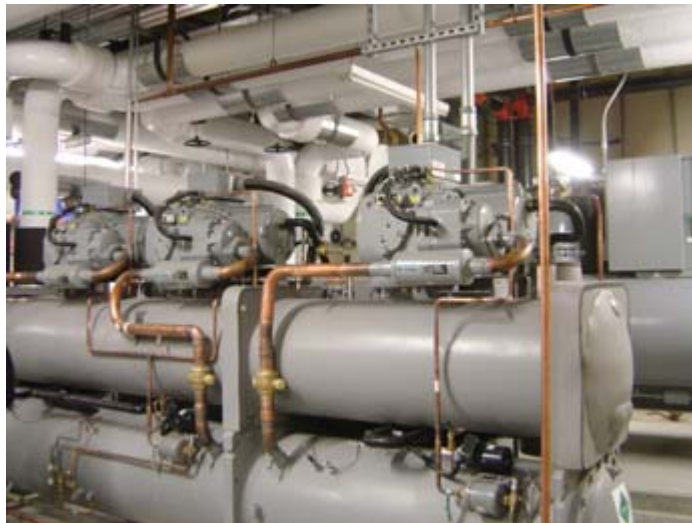
The Boiler Room. Don't tell me we ignore the "pretty" parts!
