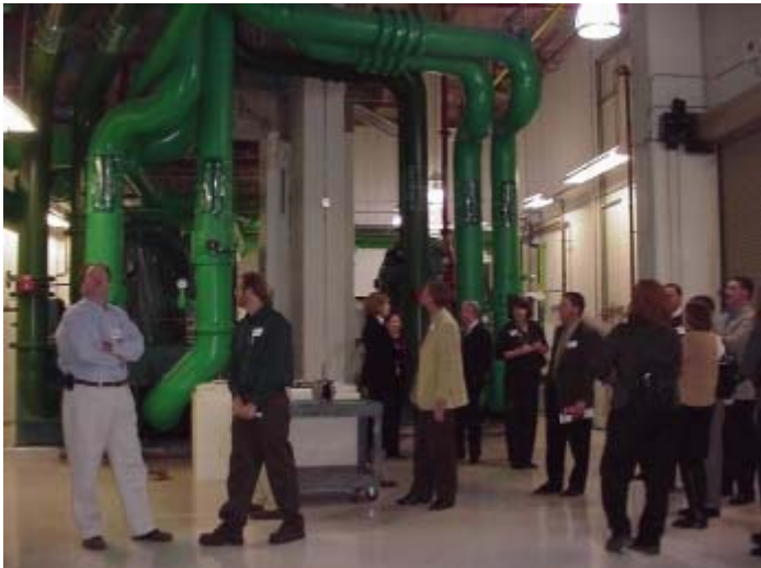
Only IFMA members got the tour of the boiler room!
